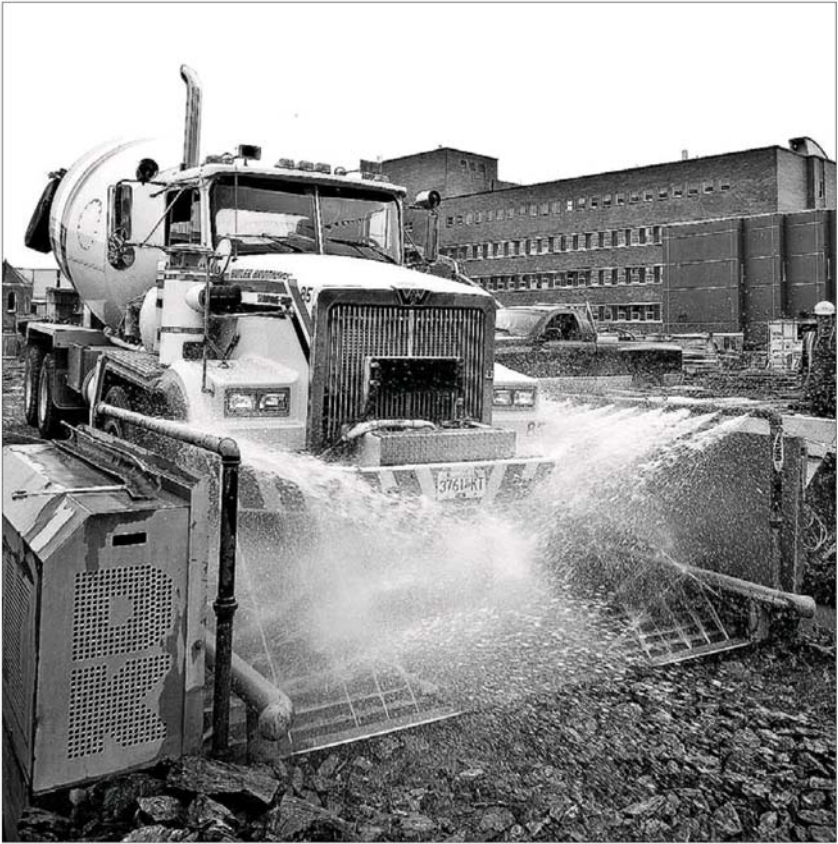
DEBRA BRASH, TIMES COLONIST Trucks going out of the construction site at Royal Jubilee Hospital are using a wheel-washing device that is designed to reduce the amount of dirt carried onto city streets and into the air. It's part of an overall plan to cut the impact of construction on the neighbourhood.
